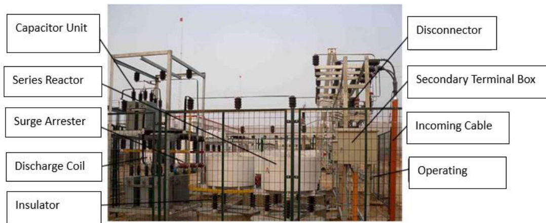
Figure 3.1 On-site Wiring of High-voltage Shunt Power Capacitor Complete Set
